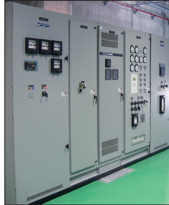
Synchronous Condenser switchgear line up
