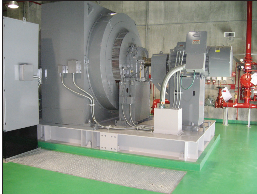
Synchronous Condenser installed in Japan
