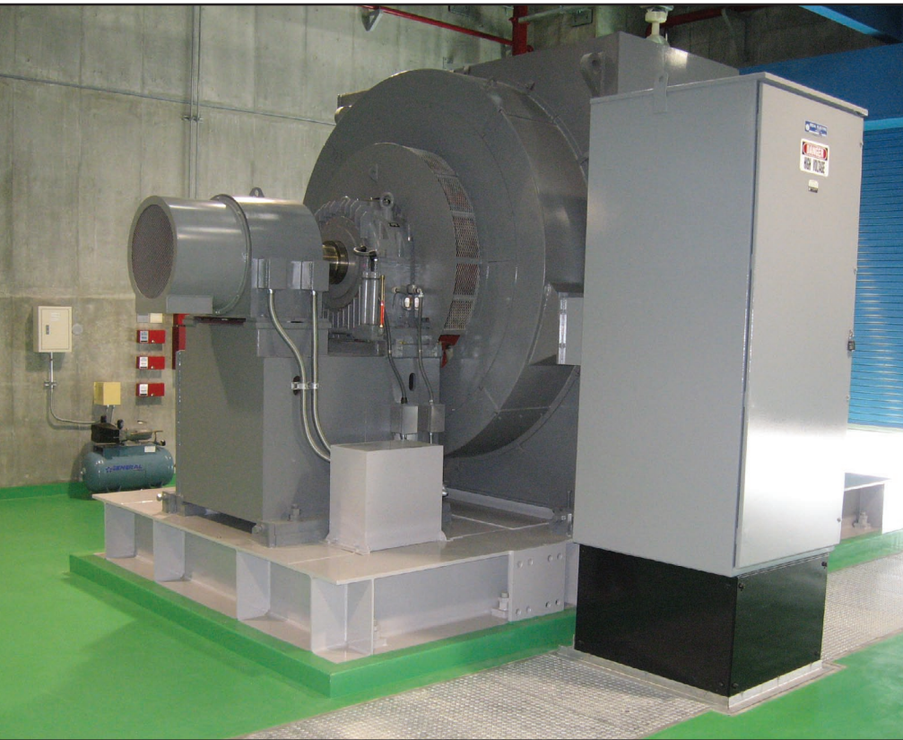
15 MVAR Synchronous Condenser
