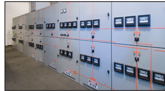
Medium Voltage Switchgear
