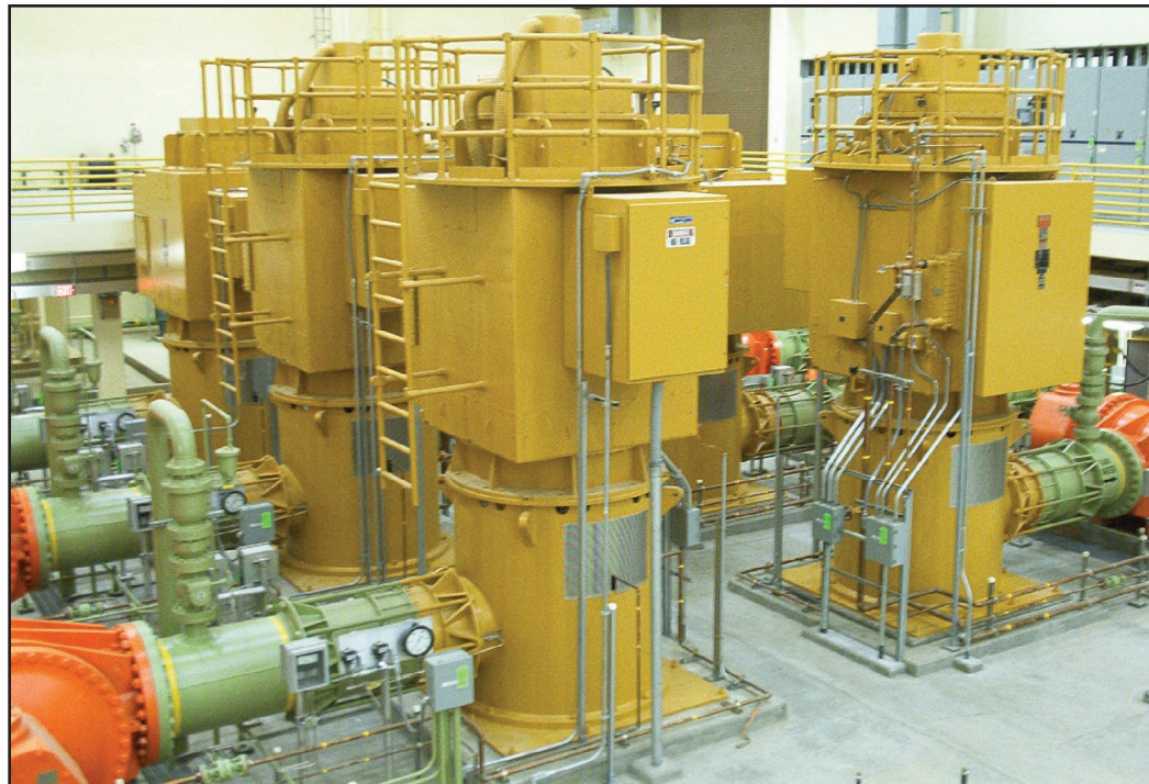
4500 HP, 720 RPM, 13,800 Volt Vertical Synchronous Pump Motors
